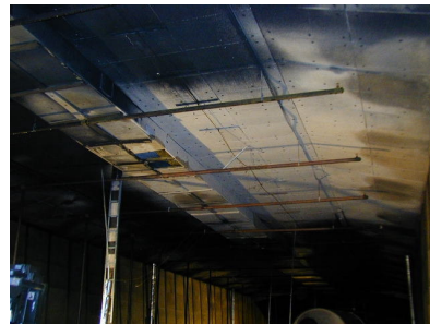
Sprinkler pipes and heads
